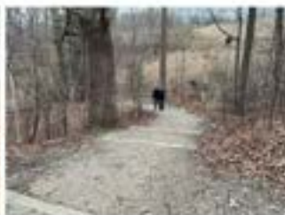
TRAIL EXCEEDS MAXIMUM ADA ACCESSIBLE SLOPE
